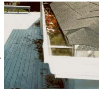
Clogged rain gutters
